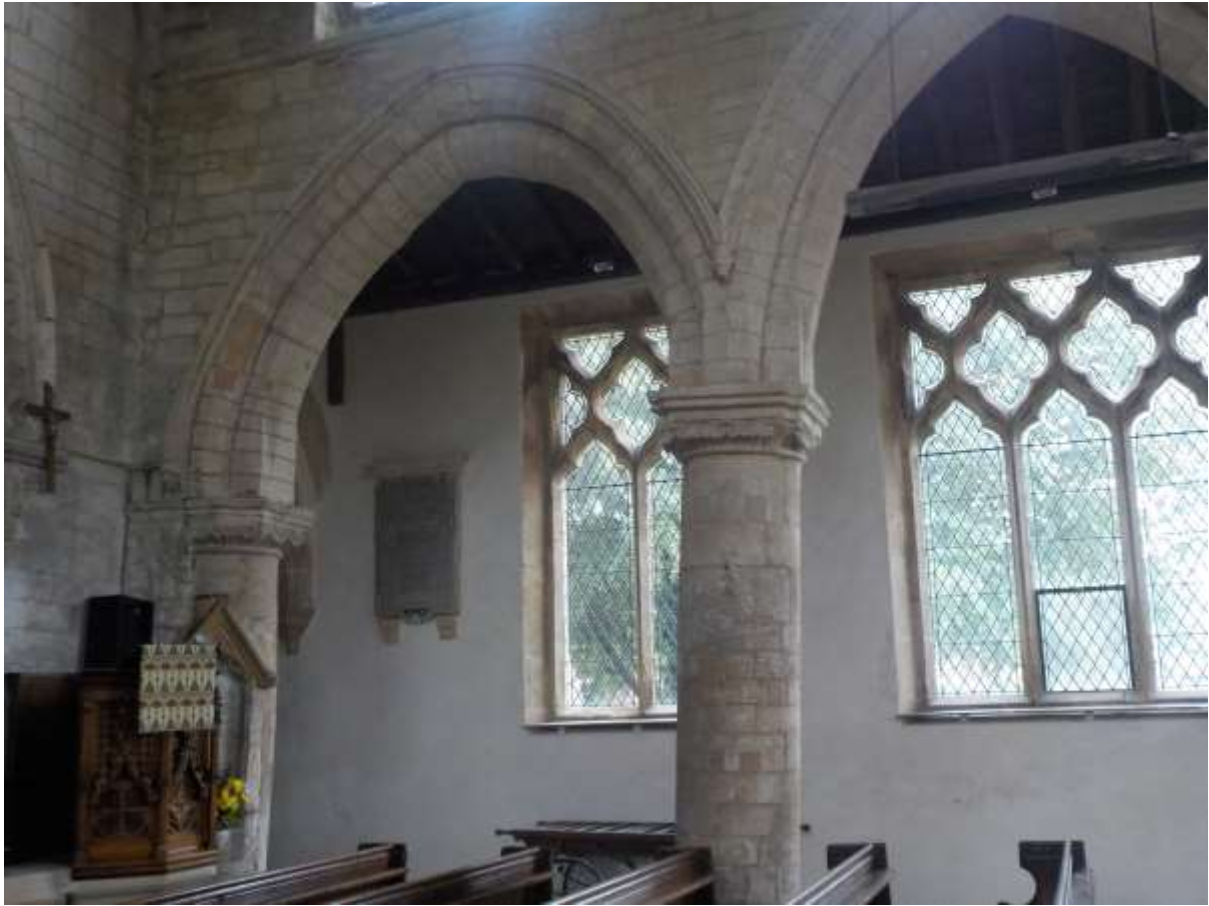
Figure 1 Leaning pier and the extraordinary arch at the east end of the south nave.
