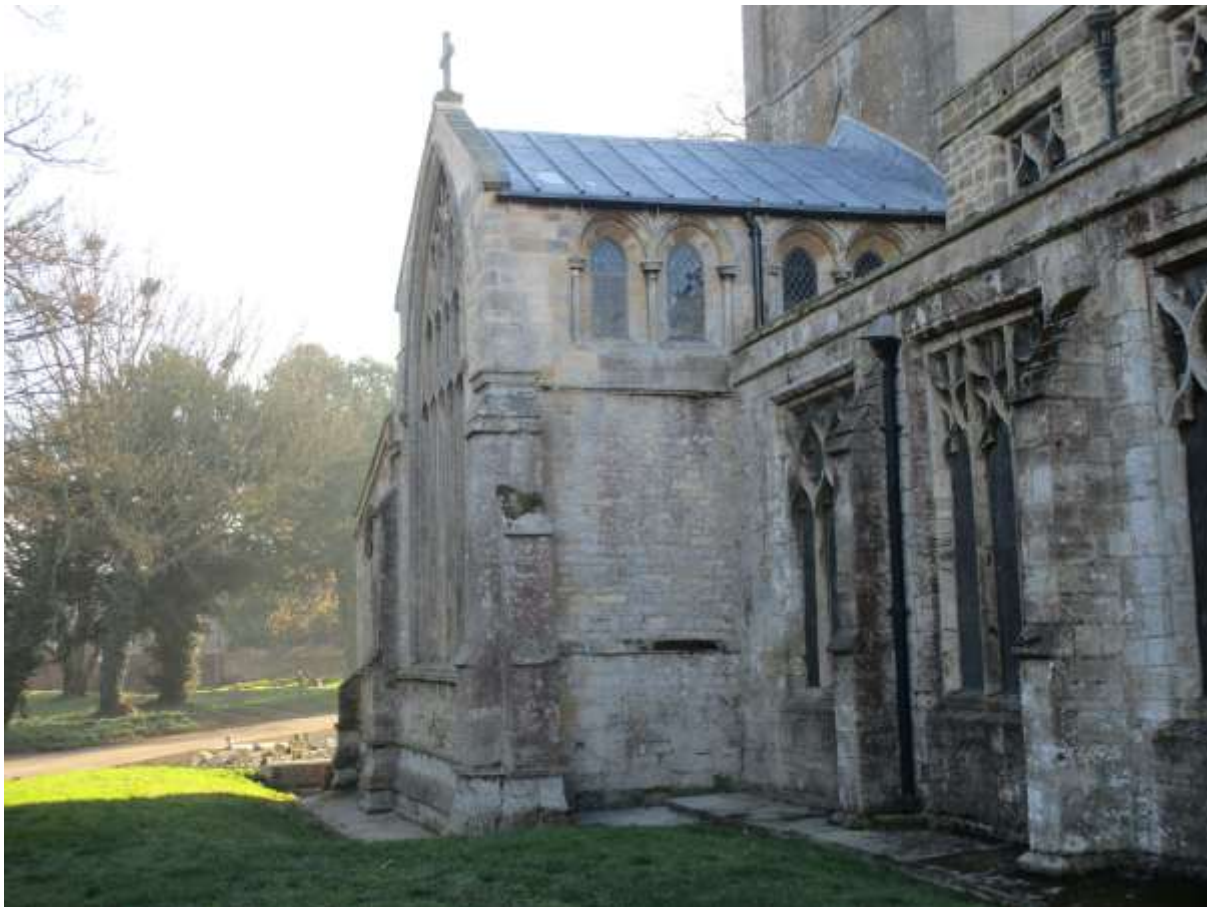
Figure 5 West side of north transept after repairs showing the new roof and repaired masonry.
